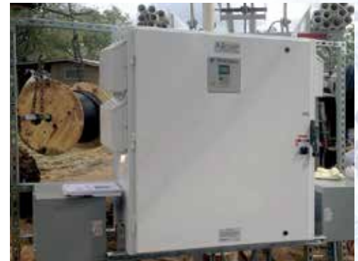
20 HP Submersible Pump Control for Irrigation.
