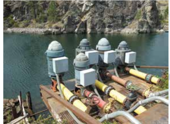
Quadplex River Booster System.
